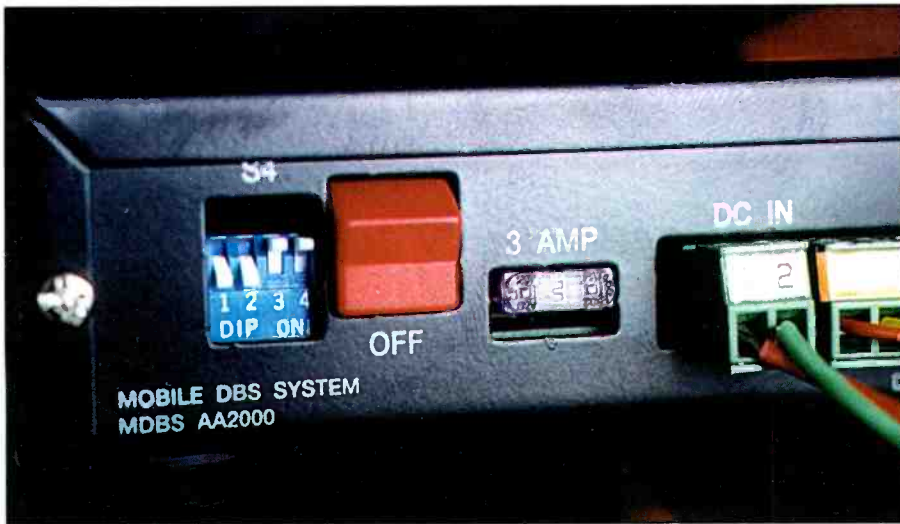
These simple DIP switches on the controller may select any or all satellites to be tracked.
